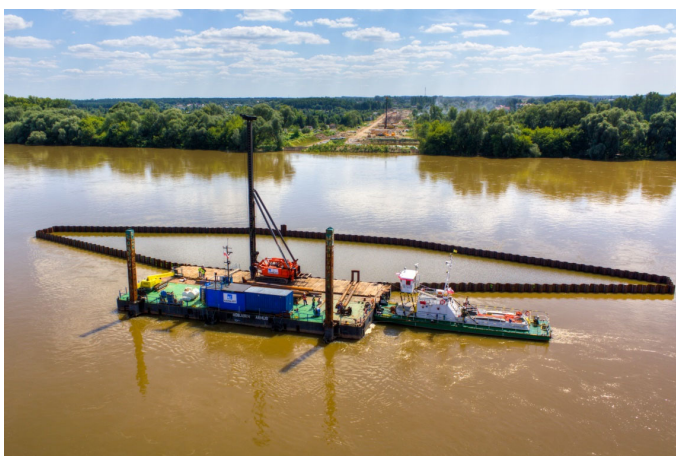
Fig. 5. "Closing" the perimeter of the island. Island steel perimeter. Floating rig with stilt supports, tugboat and vibratory pile driver.
